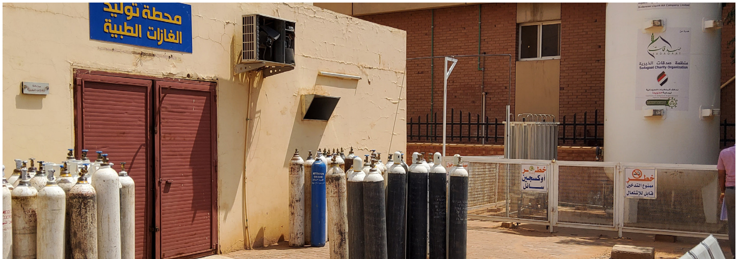
WHO team assessing the oxygen systems installations: liquid oxygen vessels with vacuum insulated evaporator (VIE) system on the right, medical gas room on the left, hosting PSA plant, vacuum system and high-pressure oxygen cylinder distribution ramp. Photo credit: WHO/Hugues Gaertner.
