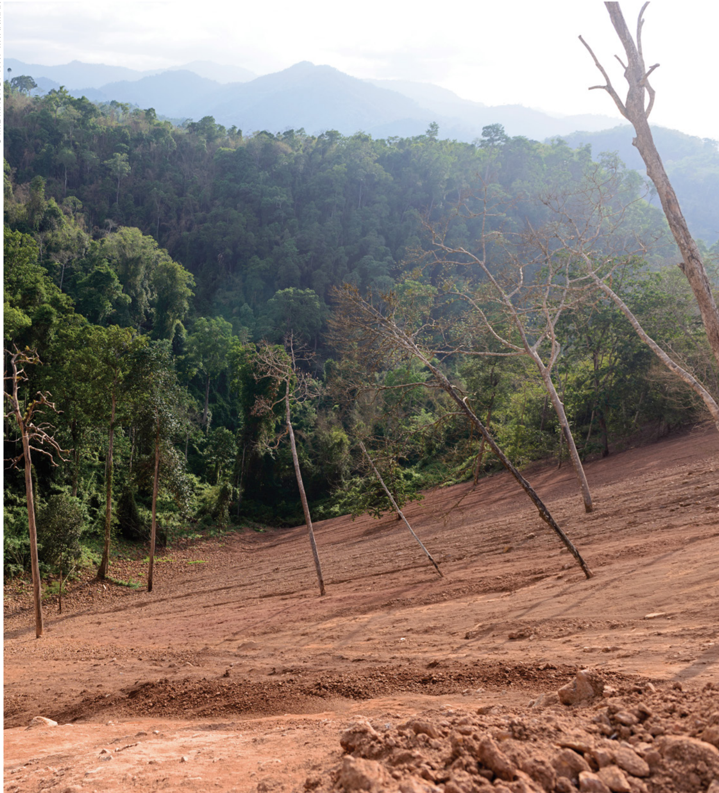
Slopes along the access road for the planned Dawei road on Elephant Cry Hill.
