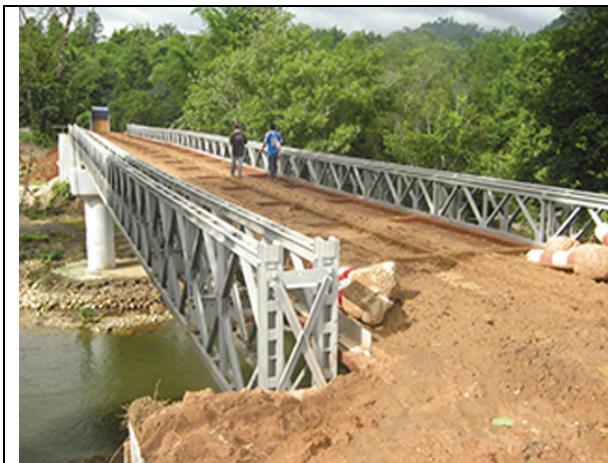
The photo above was taken on December 30 th 2012 in C--- village, Kawkareik Township, Dooplaya District/Southern Kayin State. It depicts the construction of a bridge by the Myanmar government in an attempt to try and improve the lives of the villagers. The construction destroyed the villagers' plantation fields and they reported that they were given insufficient compensation. [Photo: KHRG]
