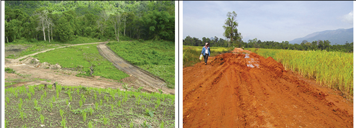
The photo on the left was taken on July 30 th 2013 in L--- village, Kawkareik Township, Dooplaya District/Southern Kayin State. The photo shows the preliminary stage of the construction of a road which destroyed villagers' paddy fields. Villagers reported that they were not provided with any compensation for damaged land. The photo on the right shows a paddy field in N--- village, Kawkareik Township, Dooplaya District/Southern Kayin State in 2014. The Thoo Lei Company previously constructed a road through this paddy field. The road is now being reconstructed again and has blocked an irrigation ditch causing the surrounding paddy fields to flood. [Photos: KHRG]
