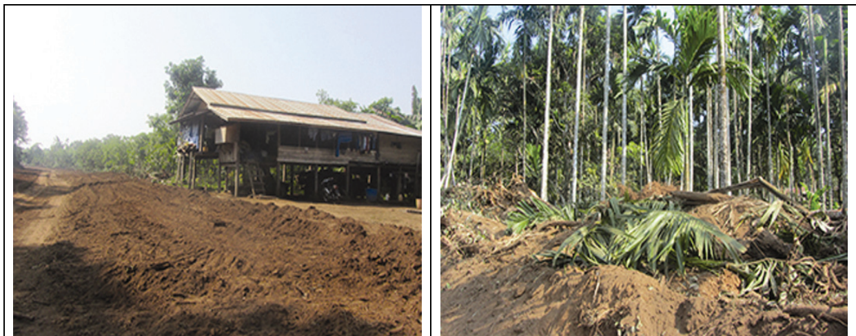
These photos were taken on December 10 th 2013 in H--- village, Kyonedoe Township, Dooplaya District/Southern Kayin State. The first photo shows road construction which damaged villagers' lands and destroyed villagers' home compounds. The second photo shows a villager's betel nut plantation that was destroyed as a result of the road construction. The villagers reported that they were told they would receive compensation, however, they are yet to receive any. [Photos: KHRG]
