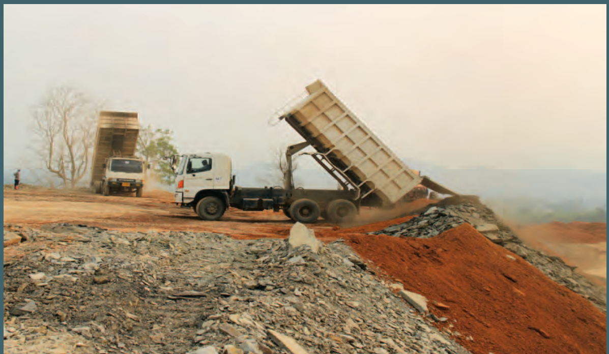
Mining waste is simply dumped in large piles at Khon Chaung Gyi mining site
