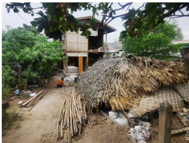
Picture 6. Collapsed animal shelter in Sagaing Tsp, Kyauk Tar VT, Kyauk Tar village (Sagaing)
