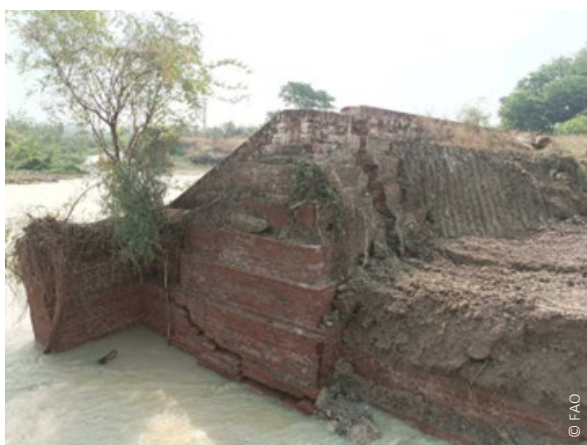
Picture 1. Collapsed retention work in Shwebo, Kanthar Kone village (Sagaing)
