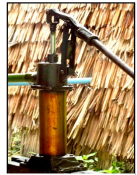
Figure 3.10.4-d - A rusted hand-pump due to high iron in delta
