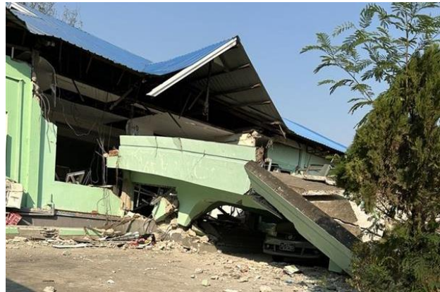
Collapsed health facility building in Nay Pyi Taw (©WHO Myanmar)
