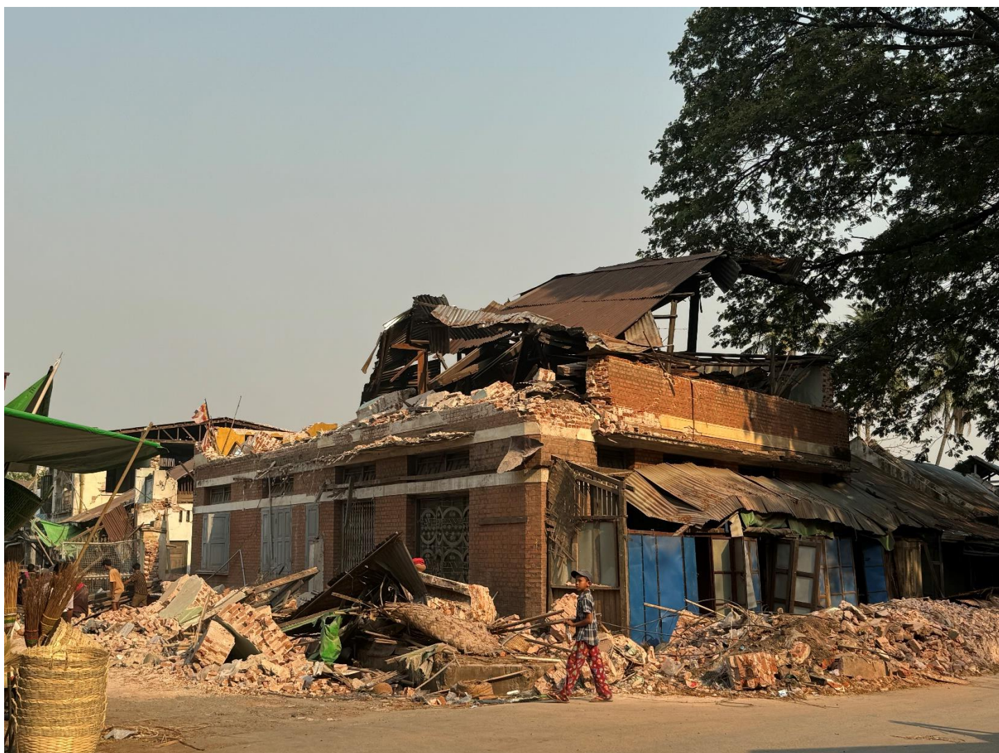
Photo: A heavily damaged building in Nay Pyi Taw. Credit: OCHA/Christina Powell
